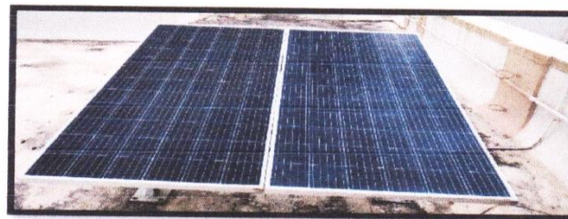
Solar Panels on the college roof top
